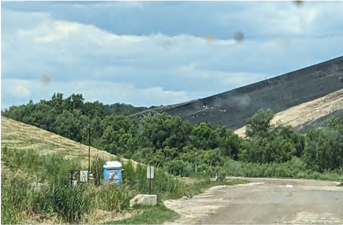
Plastic cap and geocomposite awaiting more clay on West slope on masss
