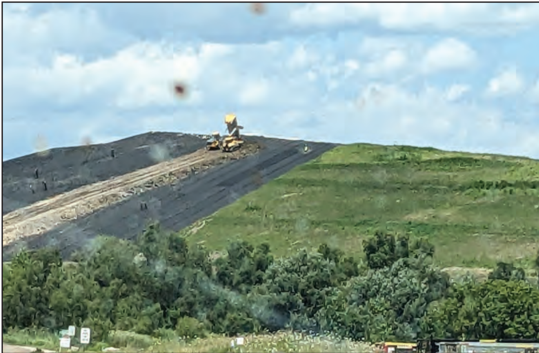
Plastic cap and geocomposite awaiting more clay on West slope on mass
