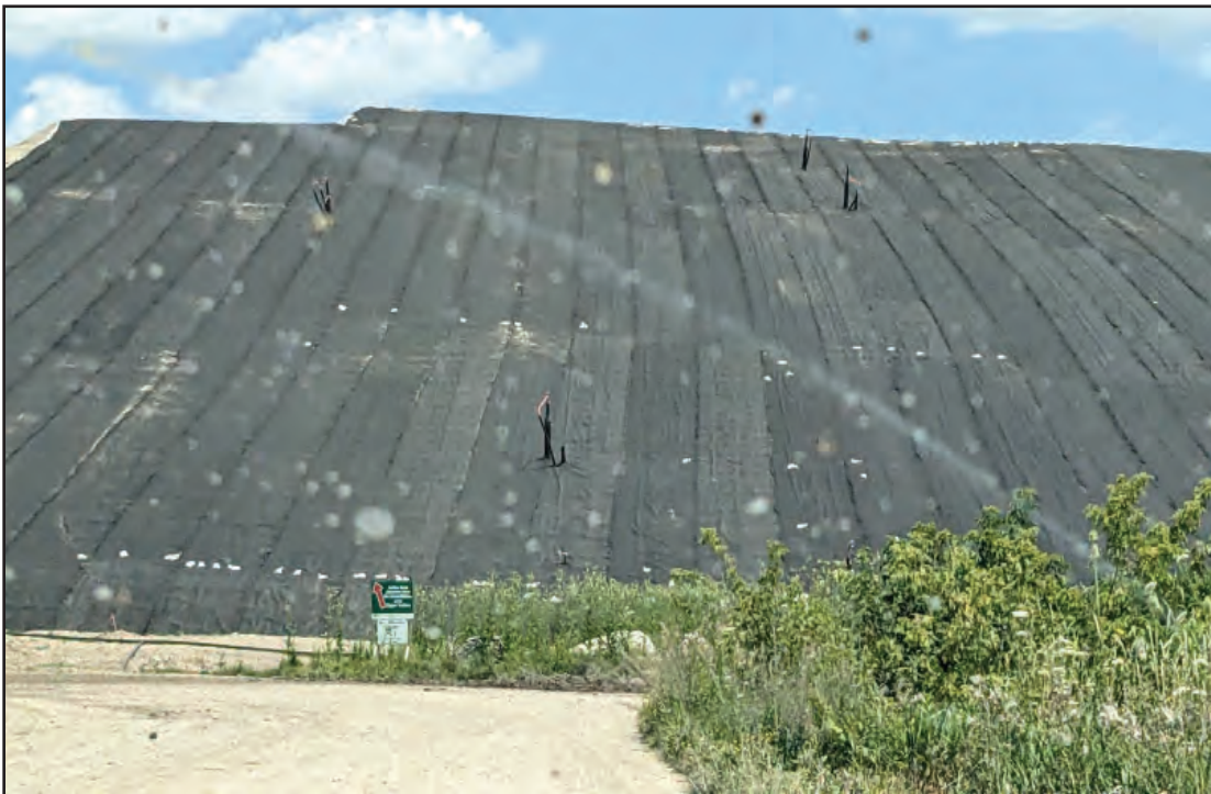
Plastic cap and geocomposite awaiting more clay on West slope on masss
